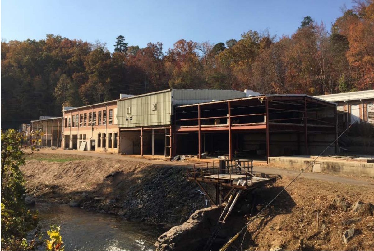
East wing of Tryon Hosiery Mill, view to southwest (Dam on Pacolet River in foreground)
